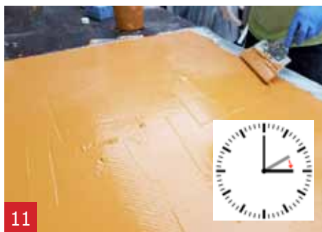
10 Apply this with the spatula on the surface of the panel to create a smooth finish layer. Let it cure for 1 hour.
