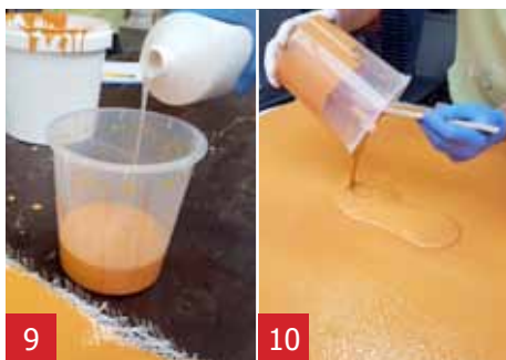
9 Add 1% of Thix A to the remaining A1 and stir well with a sturring rod. The A1 becomes thicker.
